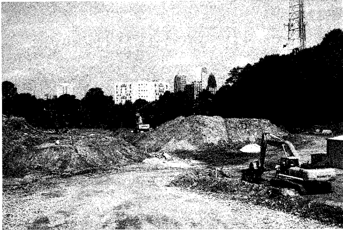
Taken through the construction entrance to Georgia Power's property on Ponce Place, this photo shows site preparation activity as crews work to replace a decades-old sewer line.
